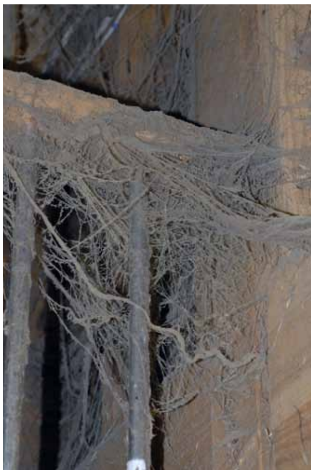
Cobwebs are extremely flammable and can spread fire easily. DUSTY PERIN PHOTO, www.dustyperin.com
